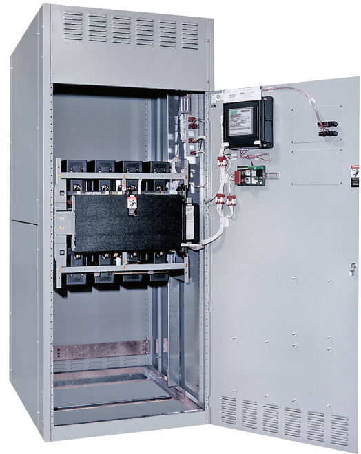
Fig. 3: Four pole, Delayed Transition 2000 Amp Transfer Switch.
